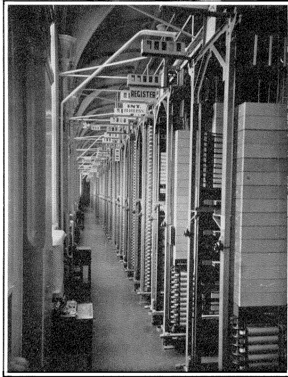
Figure 6—Teréz Automatic Exchange—Machine Switching Room, Lower Level.
